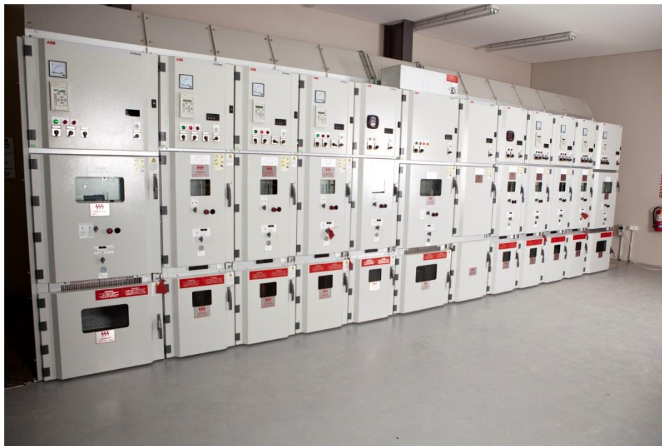
Photo 3 - Switchgear at Cloudy Bay substation
