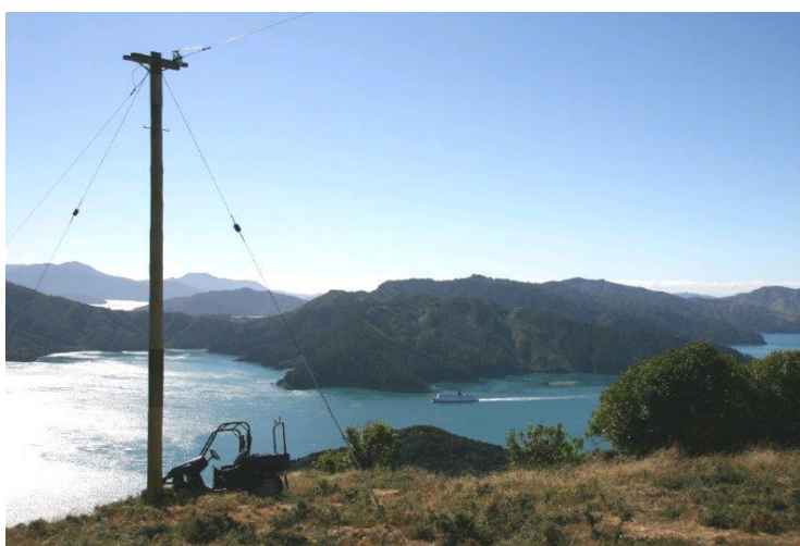
Photo 11 – SWER Lines in Tory Channel
