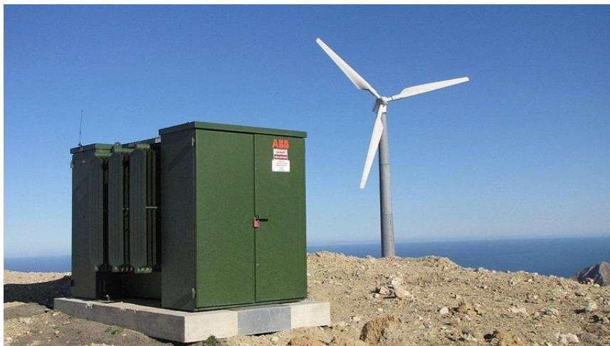
Photo 13 - 11kV Transformer at Wind farm site
