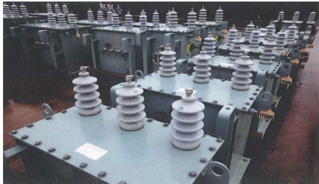
Photo 12 -- Transformers in Taylor Pass Yard
