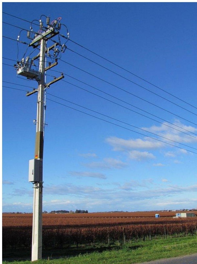
Photo 9 SCADA Controlled 11kV recloser
