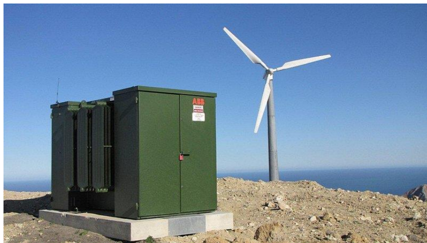
Photo 13- 11kV Transformer at Wind farm site
