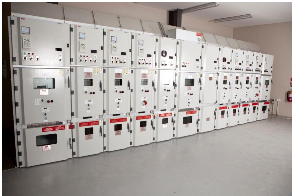
Photo 3 - Switchgear at Cloudy Bay substation
