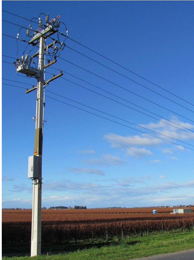
Photo 9 - SCADA Controlled 11kV Recloser
