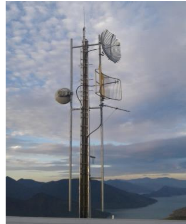
Figure 70: Communications mast at Takorika with varying antenna
