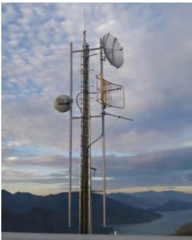
Figure 69: Communication mast at Takorika with varying antenna
