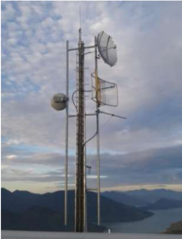
Figure 69: Communications mast at Takorika with varying antenna
