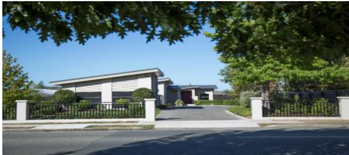
Figure 11: Photograph of ML's 33kV Waters zone substation
