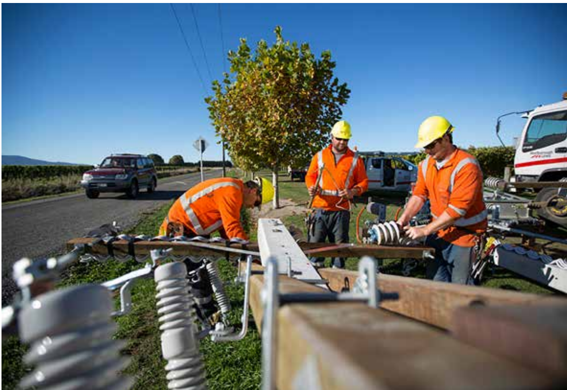
Network investment is ongoing.
