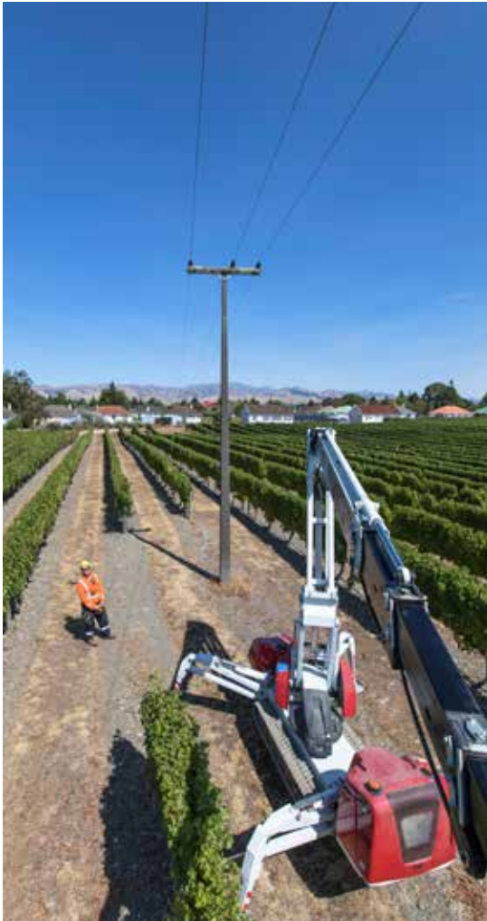
OUR DINO TRACKED EWP ENABLES ACCESS TO OUR ASSETS THROUGH NARROW VINEYARD ROWS AND SITES WITH DIFFICULT TERRAIN.
