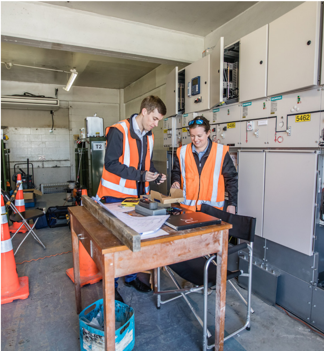
Electrical engineers, Brendan Sutherland and Irene Anderson, getting into the nitty gritty at Kinross Street substation.
