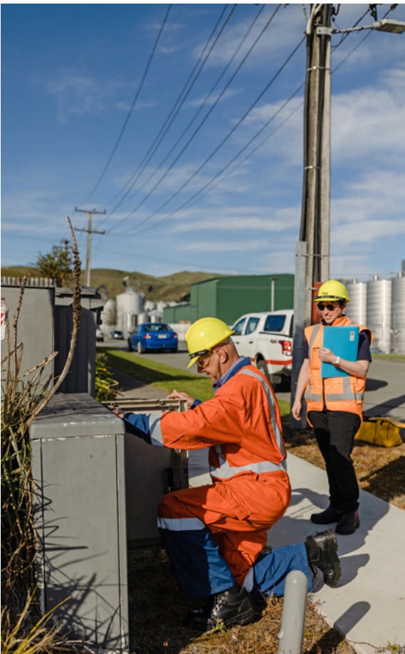
▲ Rachel McCormick and Piet Marx checking connections in a distribution pillar box.
