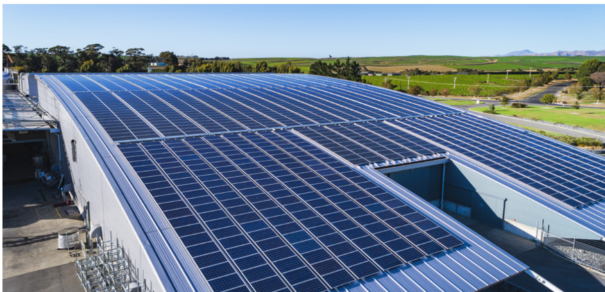
▲ Solar panels located on Yealands’ winery roof at Seaview, Awatere Valley.
