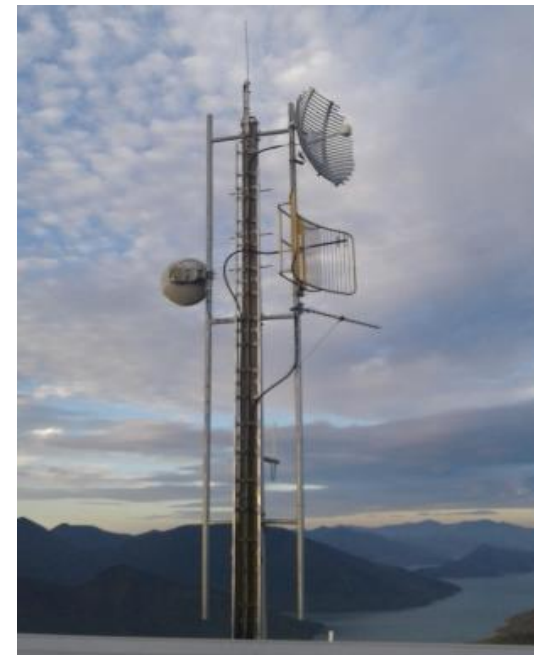
Figure 71: Communication mast at Takorika with various antenna
